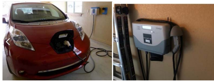
Figure 5. Nissan Leaf and charging station installed at research residence.
